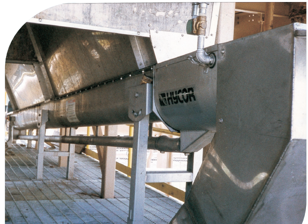
Receiving screenings from multiple pieces of equipment
